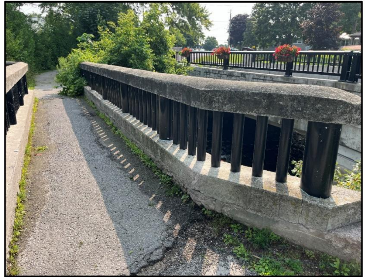
South barrier system
