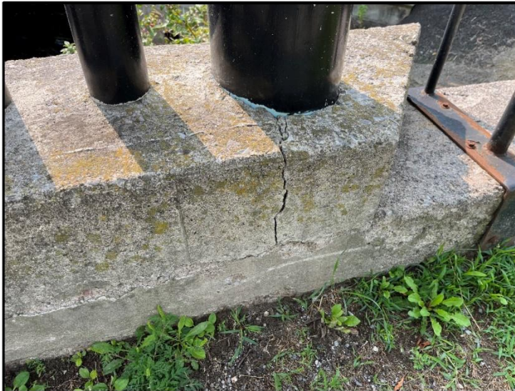
Wide crack in curb
